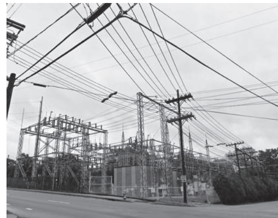
(Below) Kenilworth Substation before expansion
