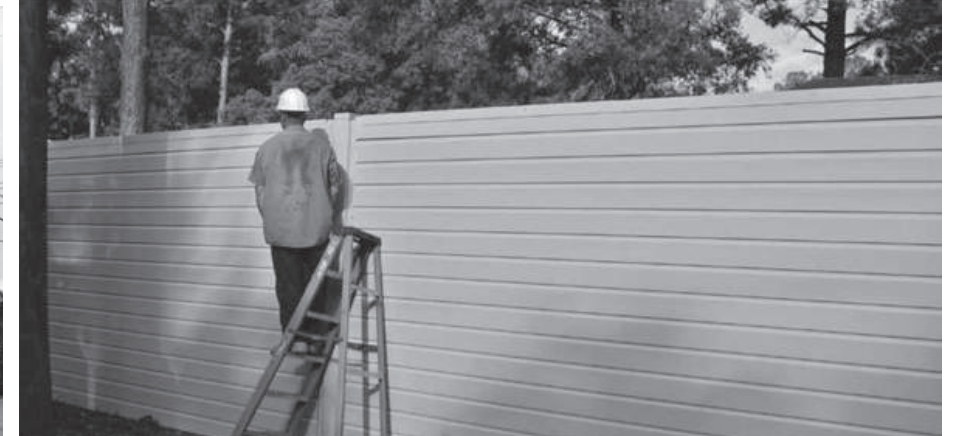
(Below) What Duke Energy is proposing as a wall (appx. 1000 linear feet!)
